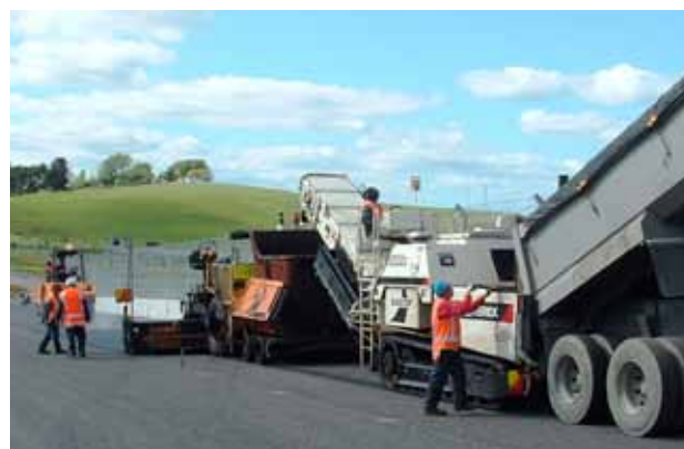
Photo 2: The innovative paving process applied for the surfacing of the Hampton Downs race track
